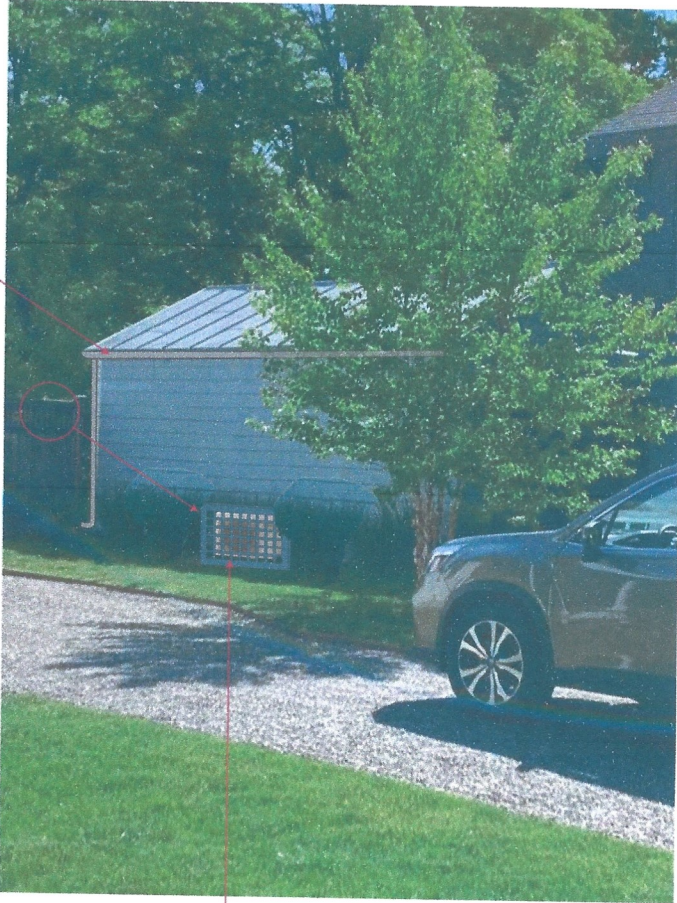
Mini split heat pump - appr 24" h x 36" w Behind 48" h x 48" w lattice screen.
