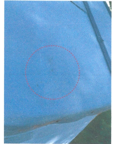
Painted-over holes on roof showing where/how former gutter was attached.
